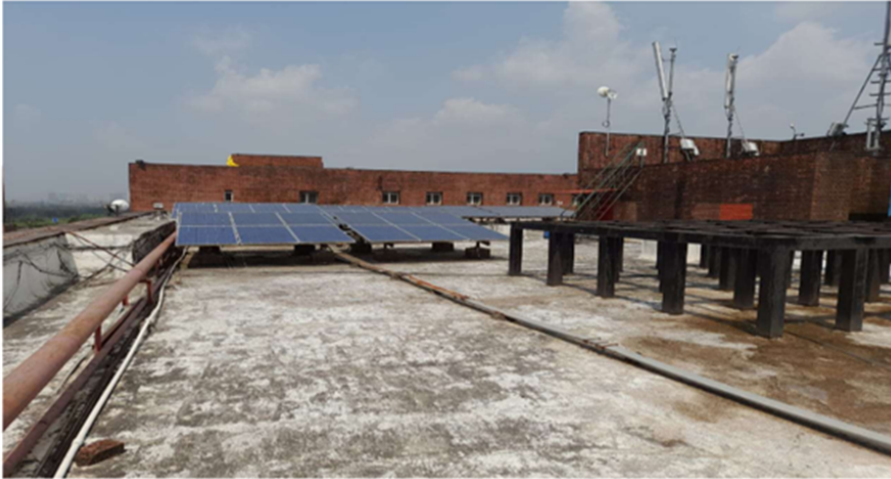
Figure .9.11.1 Solar panel setup_01
