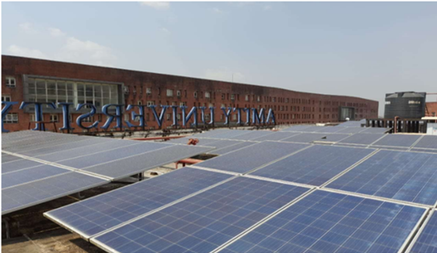
Figure .9.11.2 Solar panel setup
